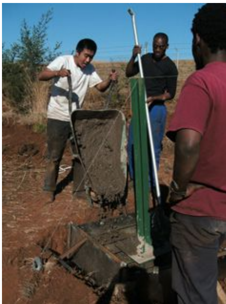
UROP student Peter Lu '11 pours cement with mechanical engineers Motlatsi Sekhesa (center) and Tumelo Makhetha, both of whom are with STG International, a nonprofit company formed by MIT PhD student Matthew Orosz.
